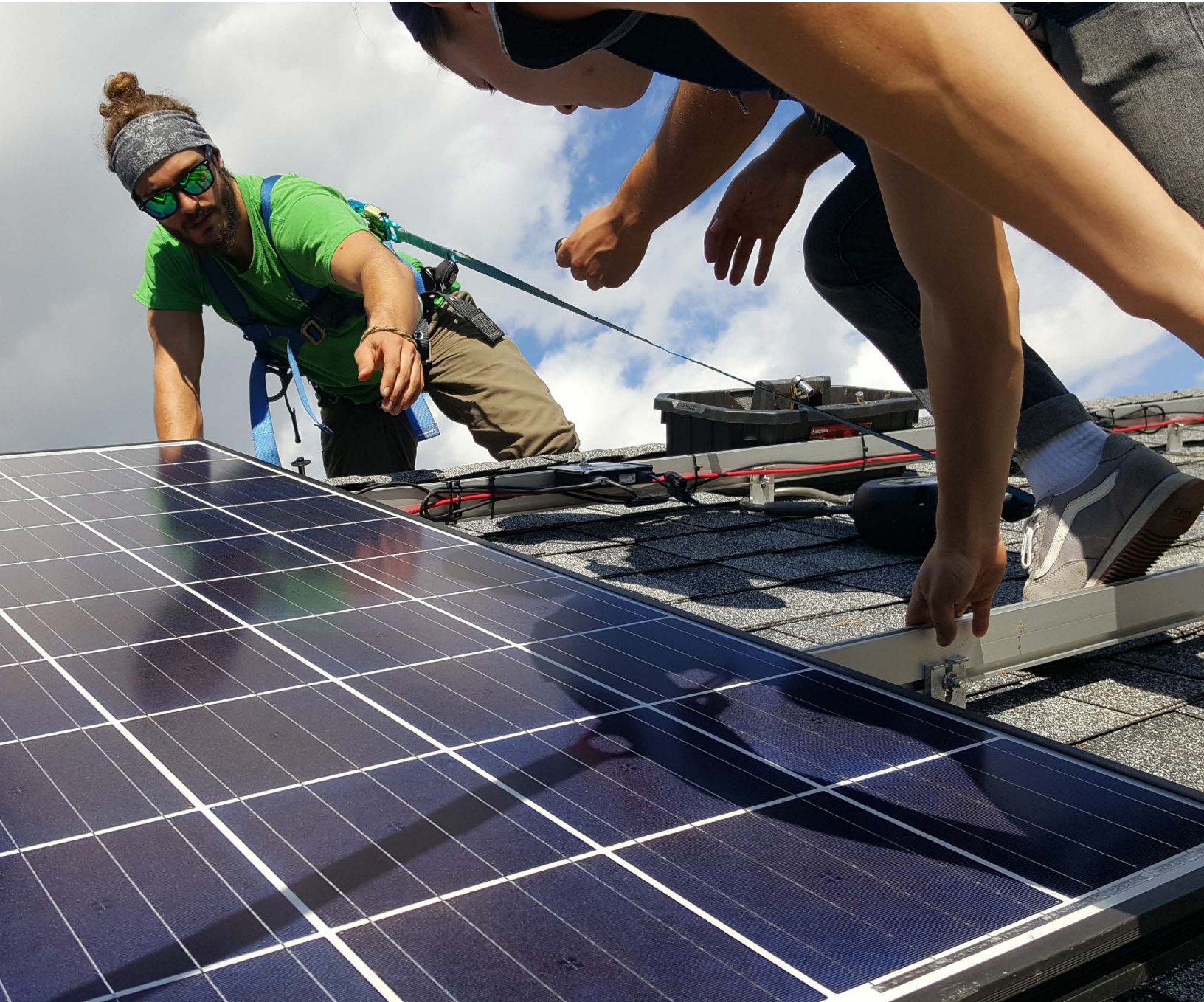
Bates College students install solar panels on the roof of the College's coastal research facility. Photo credit: Tom Twist
