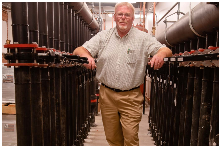
Skidmore College Assistant Director of Construction Services, Paul Lundberg poses with one of 20 geothermal nodes at Skidmore College.
