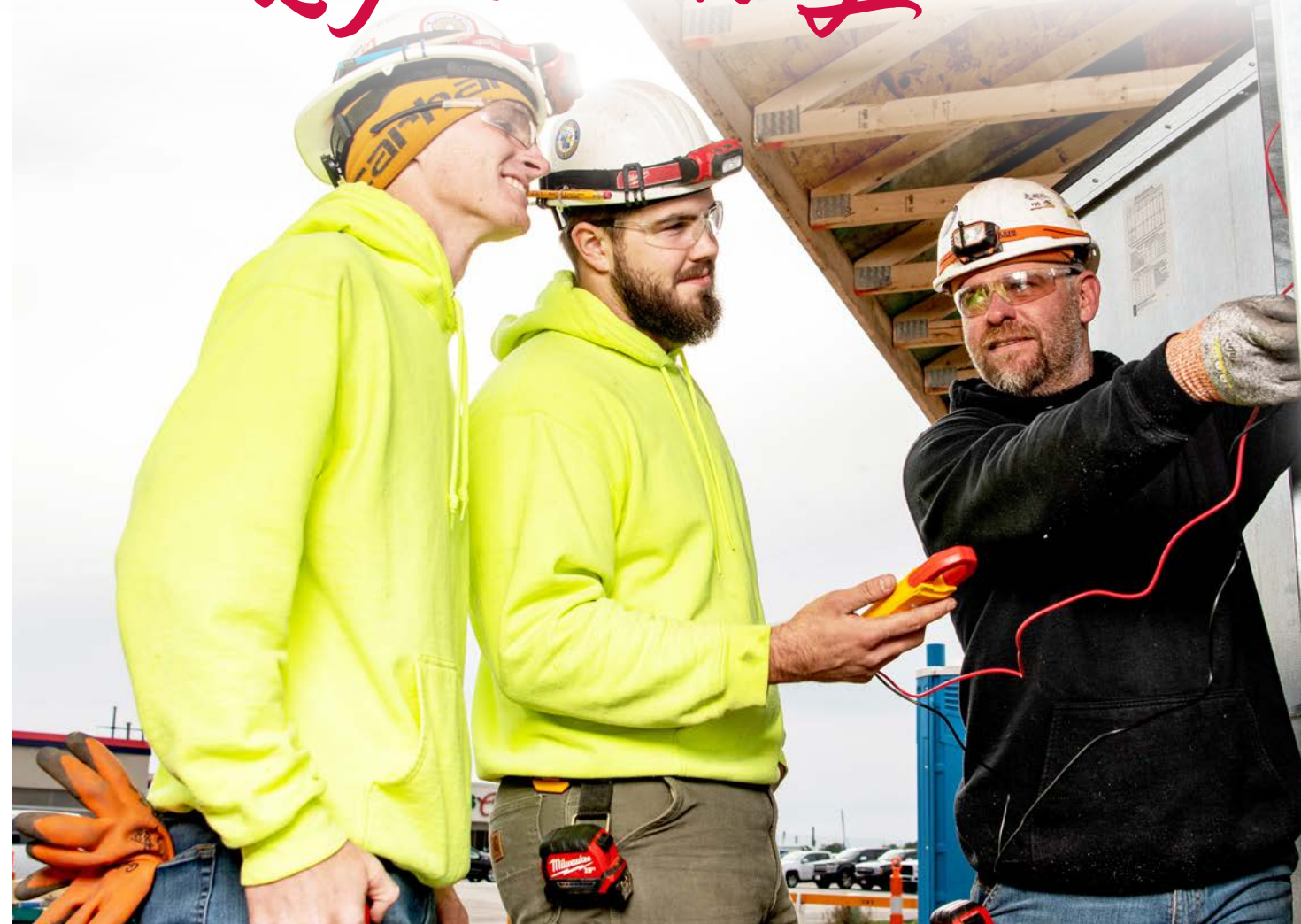
Two apprentices from Kish & Sons Electric receive training on the job site.
